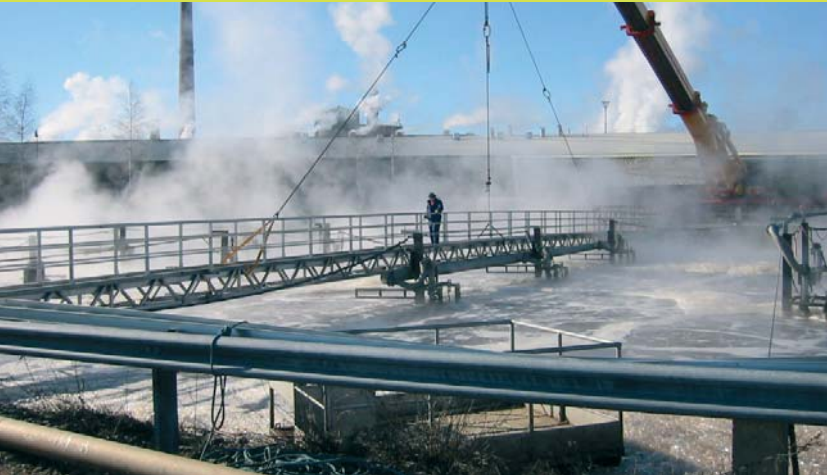
Industrial wastewater treatment in Kotka, Finland
